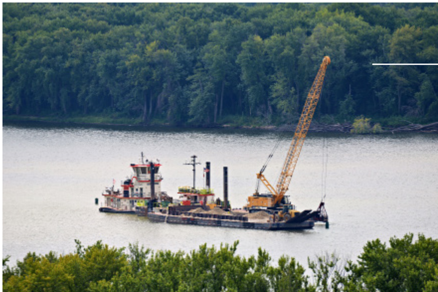
The U.S. Army Corps of Engineers working to deepen the main channel on the Mississippi river.
