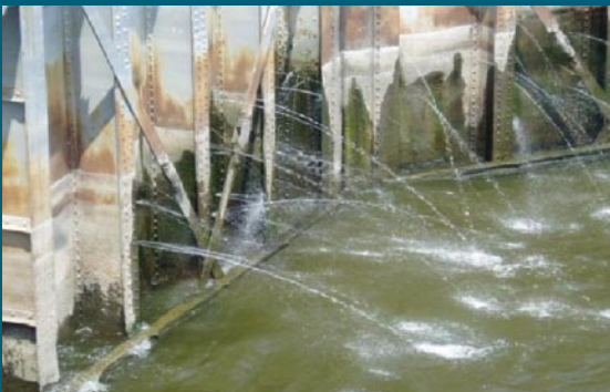
Failure of miter gates, shown here, disrupts navigation for extended periods.
