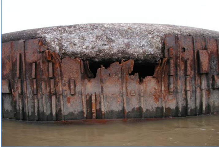
Figure 4. Cell Wall Oxidation at L&D 52. If the river should rise a few feet before the hole in this cell were repaired, it could lead to total cell failure and even lock closure. Is this type of oxidation occurring below the water line, and to how many of the cells is it occurring?
