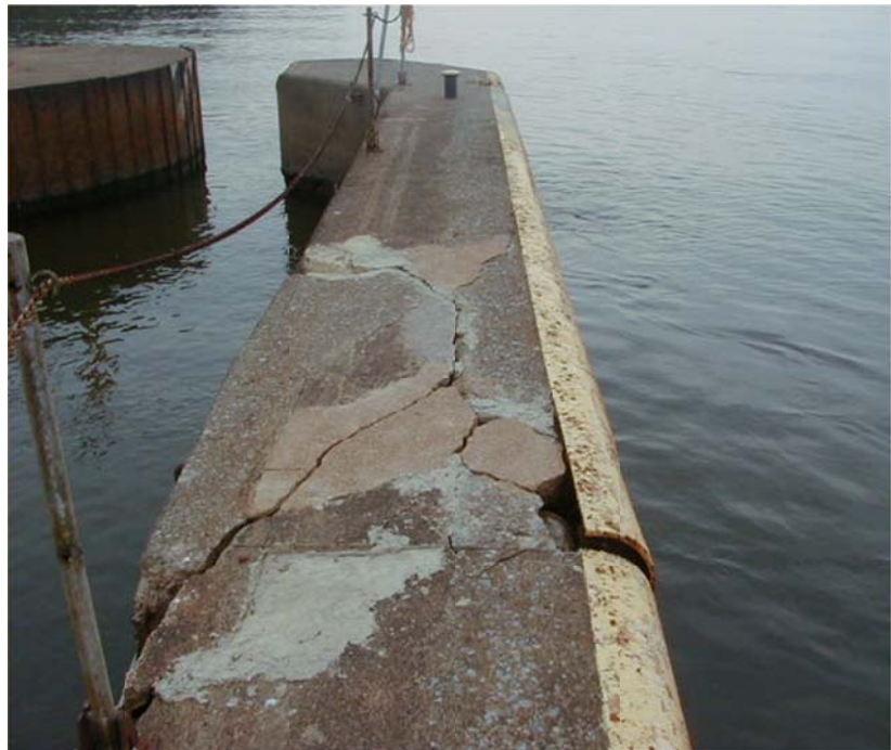
Figure 5. Approach Walls Deteriorating. How deep are these cracks, and what would it take to fix them? How long could traffic be stopped? How many cycles of cold weather and freezing rain can this wall withstand? The Corps does wonderful repair work every day, but can we expect miracles forever?
