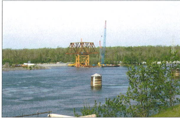
Crane work progresses April 25 on a 200-foot truss as part of moving Paducah & Louisville Railway below Kentucky Dam to make room for the new 1,200-foot lock. Funding has delayed the start of actual lock construction.
