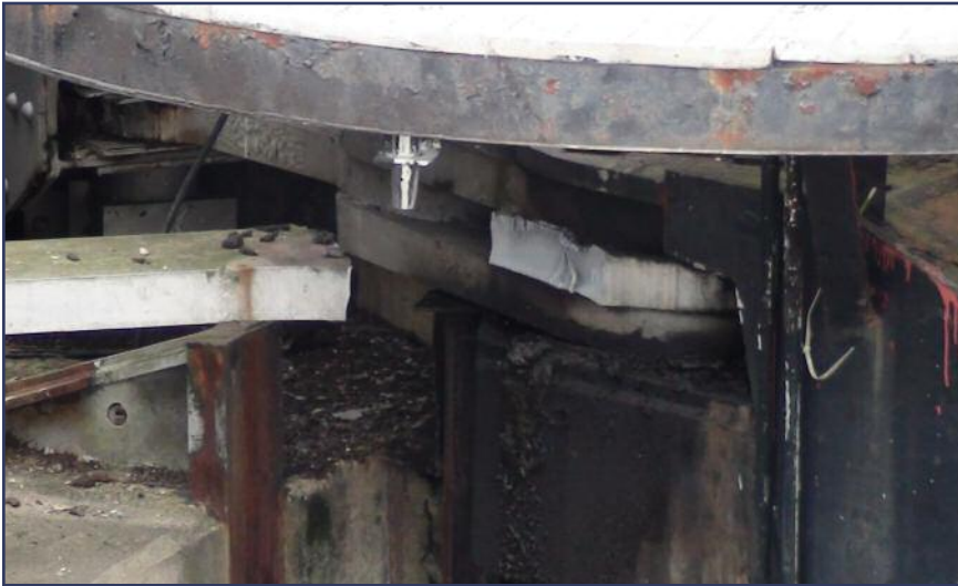
Break caused lock failure. This is the steel anchorage bar, about 4 inches thick and 12 inches wide, which snapped at Greenup Lock and let the heavy miter gate leaf fall, stopping barge traffic from using the main chamber.
