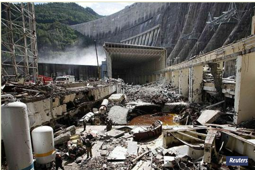
Russian dam accident. A sudden water pressure surge (a “water hammer”) ejected a 900-ton turbine in late August at Russia’s largest hydroelectric power station, which was undergoing maintenance at the time. Water flooded the engine and turbine rooms and caused a transformer explosion which claimed 75 lives. But the dam, built in 1978 on the Yenisei River in Siberia, did not fail. It is 800 feet high and 0.6 mile wide.
