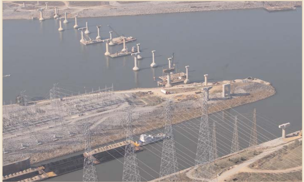
Bridge Relocations at Kentucky Lock. Before the Corps of Engineers can start construction of the downstream portion of the new Kentucky Lock Addition, two bridges over the Tennessee River have to be relocated and four large transmission towers carrying power from the dam's hydropower plant have to be moved. The bridges, each about 3,000 feet long, are for U.S. Highway 92 and the Paducah & Louisville Railway. This $185 million relocation is scheduled to be completed by 2010, about the time the upstream portion of the new lock should be finished and work begins on the downstream section.
